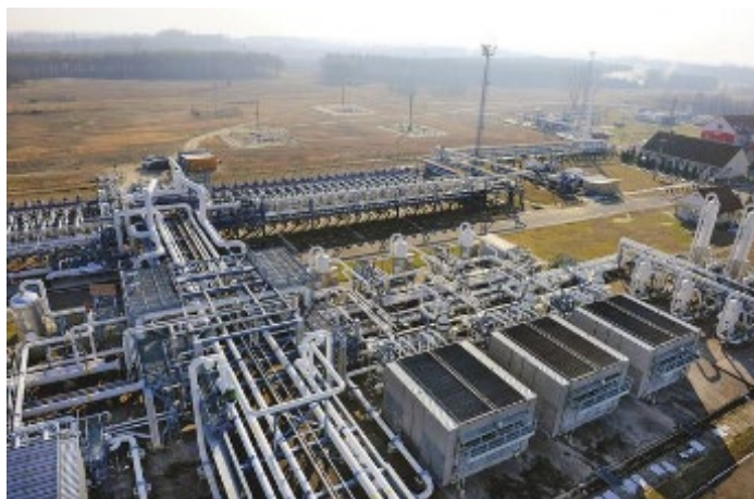
36. Figure: Natural gas pressure boosting site, Nyárlőrinc [3]
