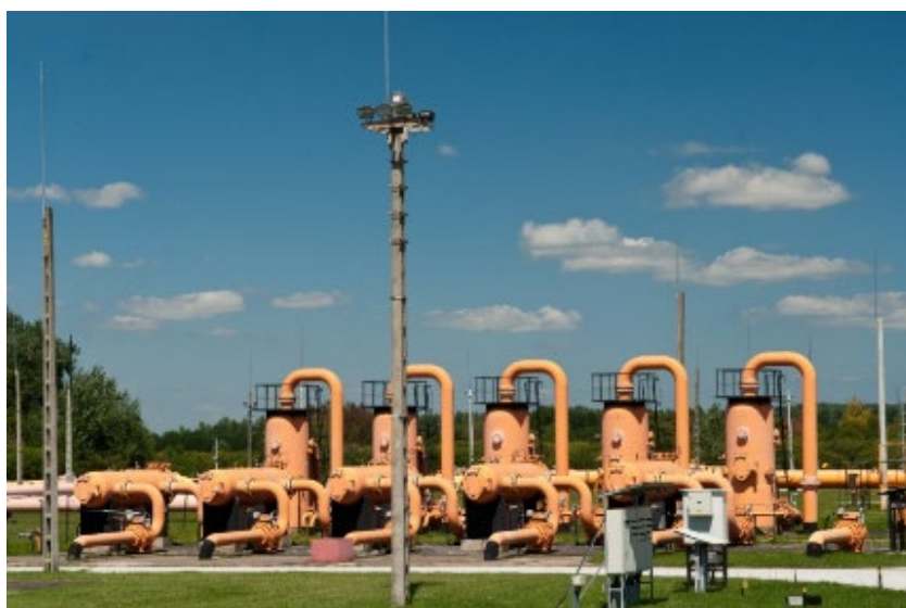
29. Figure: The first step of the pressure boosting process is the filtration of the natural gas arriving through the transmission line [3]
