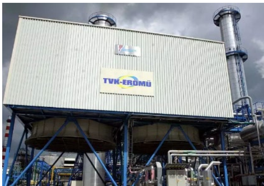
46. Figure: TVK power plant [19]
